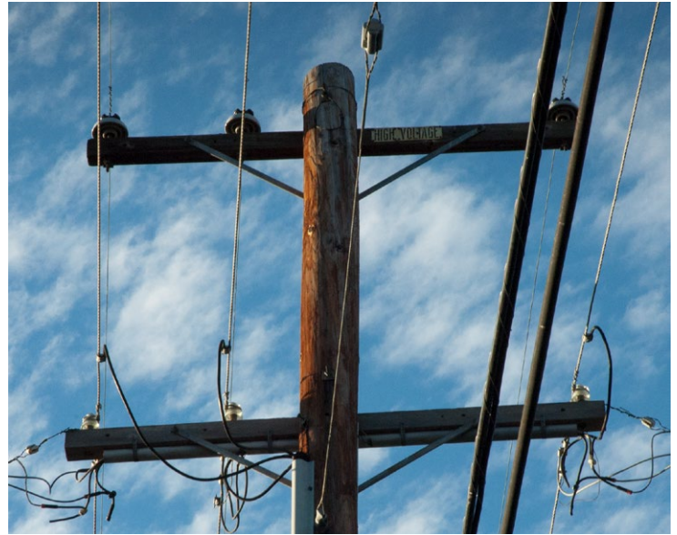
These three insulators are still working and looking good.
