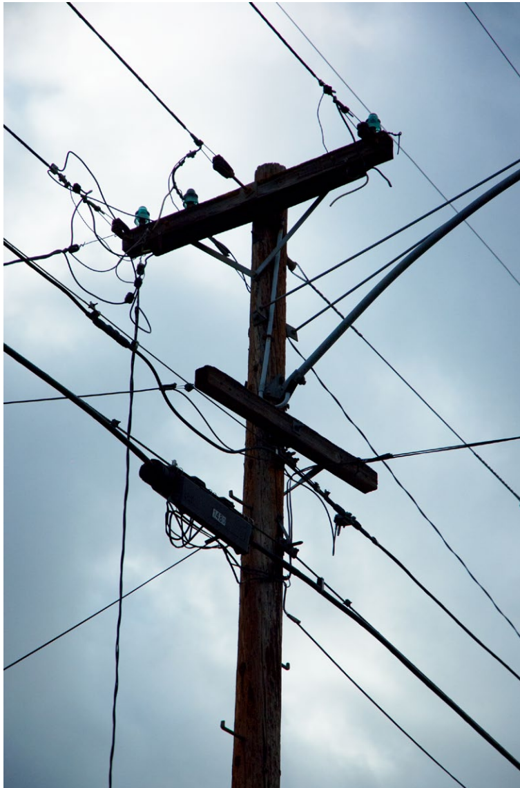
Here was a nice surprise, three aqua insulators still on duty.
