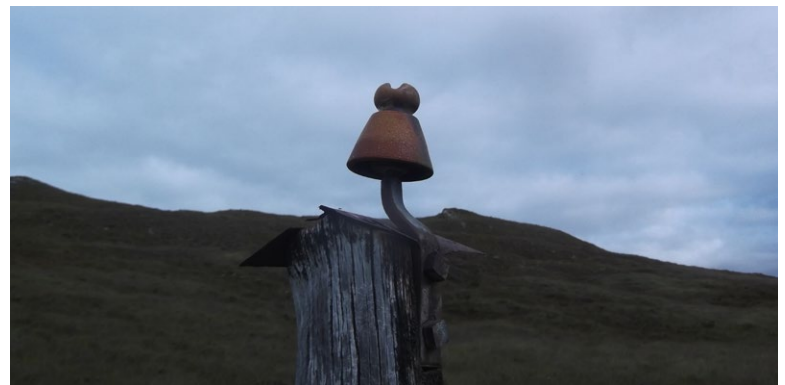
PHOTO 3 – The first Curtoys insulator we found, mounted on a very short pole.
