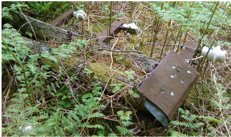
TYPICAL FALLEN 'A' POLE COMPLETE WITH INSULATORS
