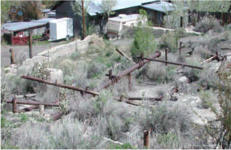
Old Steam Pipe Network in Power Plant
