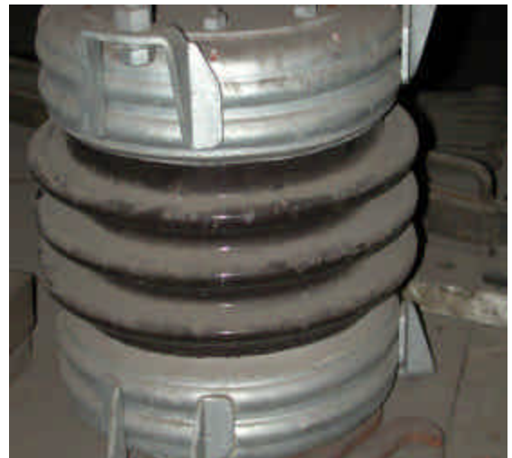
BIG Insulator! Buss bar system.
