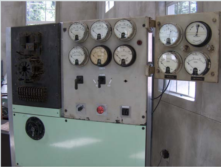
The control panel
