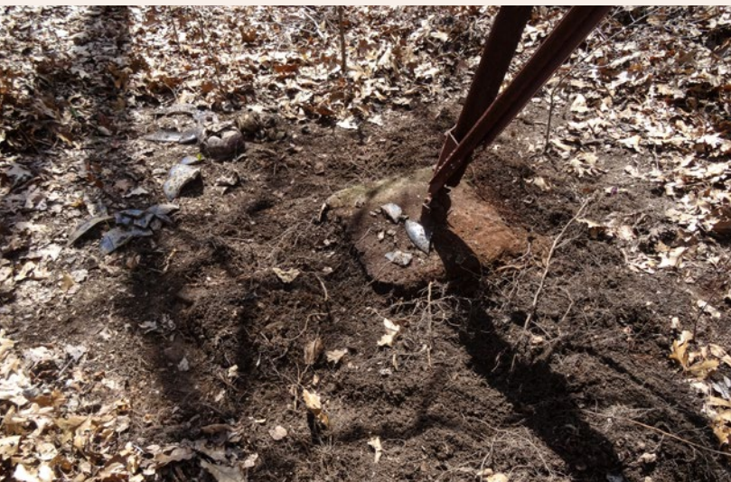
A standard cement tower footing surrounded by insulator shards.
