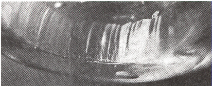
Vertical scraping lines found on the inside skirts of the 1-D insulators.
