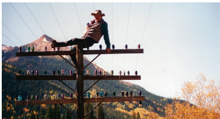
MIKE ON TOP OF ONE OF THE POLES HE CONSTRUCTED NEAR OURAY
